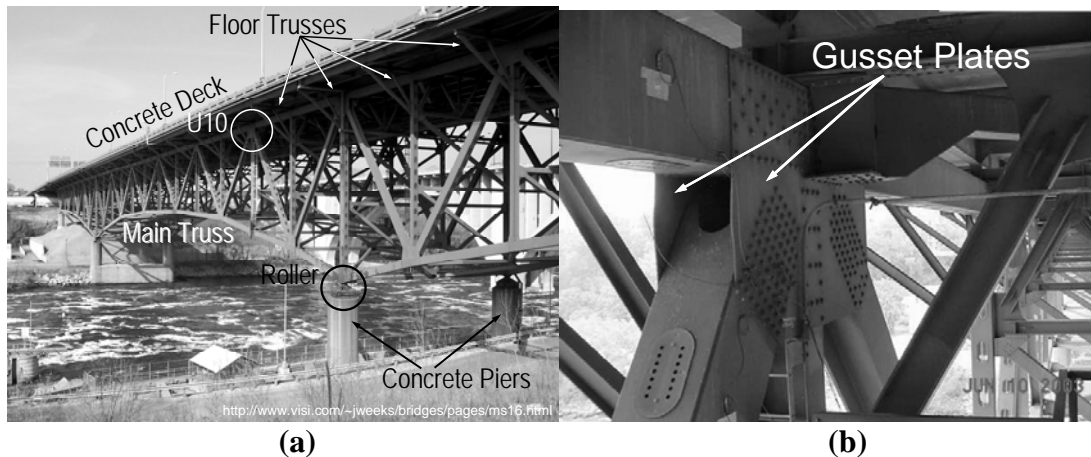
Figure 1- (a) Main structural components of the I-35W bridge, photo by John A. Weeks III ( http://www.johnweeks.com/twincities/pages/ms16.html ); (b) Close-up view of the gusset plates at the U10 node from NTSB ( Photos of I-35W Bridge, http://www.nts.gov/dockets/highway/hwy07mh024/387406.pdf ).
